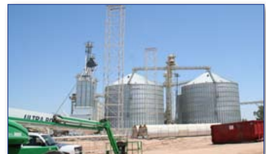
Pinal Energy uses conveyor belts to move corn from the elevator to the ethanol production facilities and to distribute the feedstock byproduct to cattle surrounding the plant.
